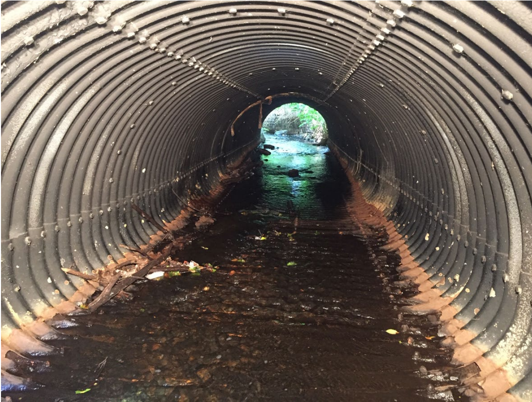
Installed 1972 - Willburgh, MA
