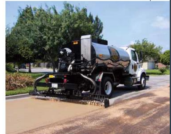
Pavement Restoration, Inc., Boerne, Tex., applies Reclamite rejuvenator to pavement in Travis County, Tex.
