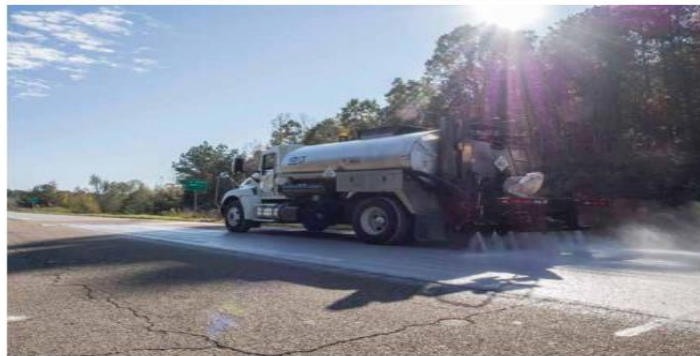
Delta Mist rejuvenator is applied to Section 53 of the NCAT Test Track.
