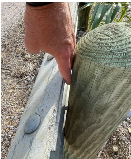
Poor beam to post connection
