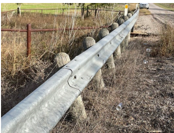
Posts leaning with no lateral support
